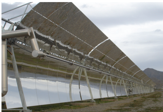
Fig. 3. Cylindrical parabolic concentrators at the PSA (Almería Solar Plant).
